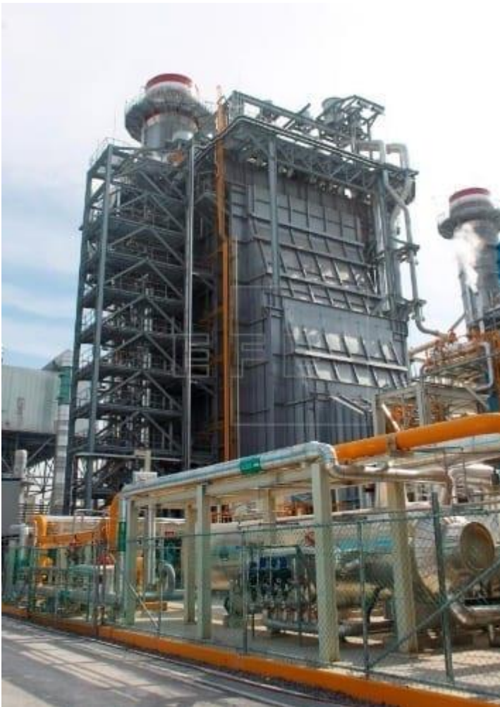
2. Wood supplied the two horizontal HRSGs, auxiliary equipment, and advisory services for the El Carmen project. Courtesy: Iberdrola S.A.
