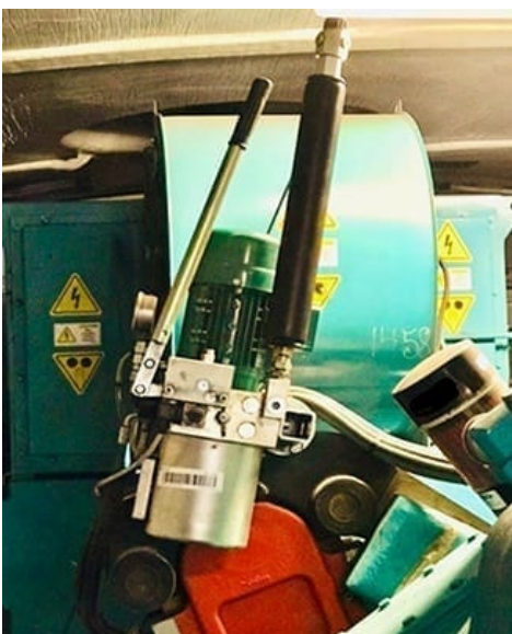
5. A piston accumulator replaced the failed diaphragm accumulator installed on the disk brake assembly shown in Figure 2. Courtesy: Parker Hannifin
