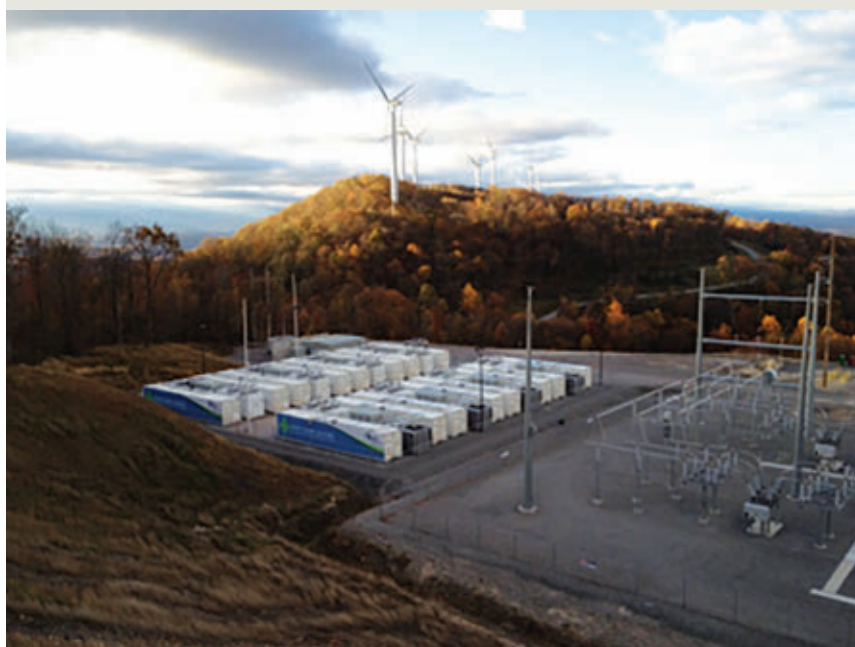
The 98MW Laurel Mountain Wind Farm uses battery energy storage to optimize energy sold into PJM and to provide regulation services.
